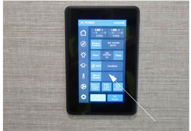
Diesel Engine Heater Switch (Located on multiplex monitor panel)
