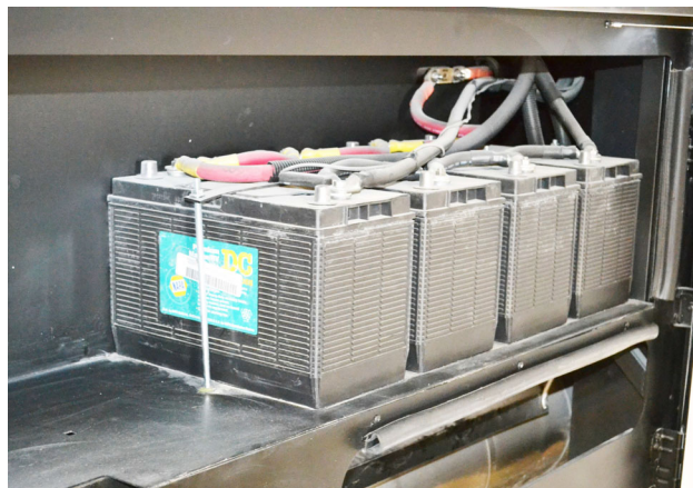
House/Coach Batteries -Typical View
